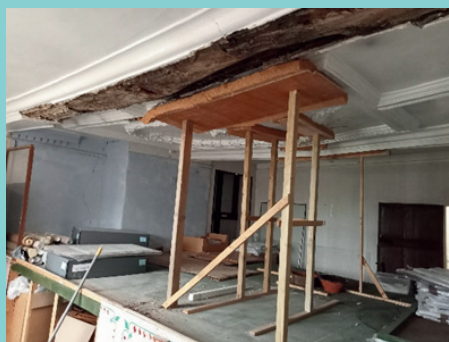
This mid 17th Century decorated ceiling will be restored to its former glory
