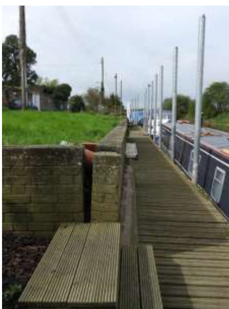
Access Steps – Rotation & Cracking
