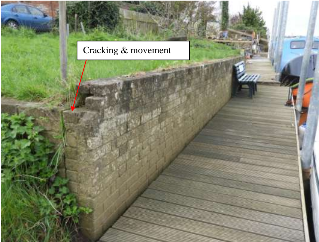
Original Landing – Cracking/Rotation RHS
