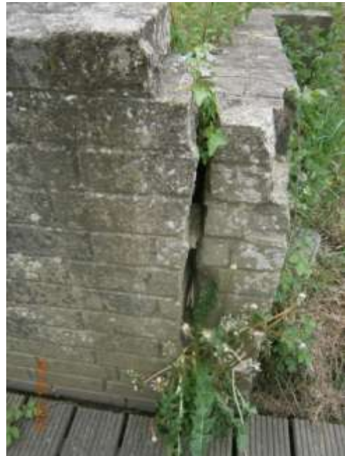
Original Landing – Cracking LHS
